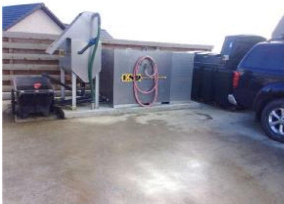
Figure 11: Investment into a closed loop wash down facility is excellent and does illustrate the Clubs commitment to investing in modern maintenance equipment.
